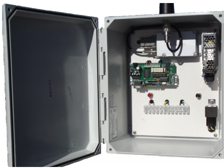
SC1 Controller W/O Battery Backup Installed
